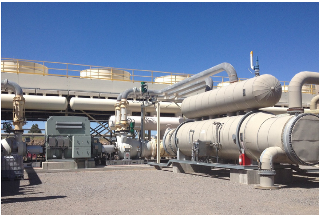
Ormat Steamboat Geothermal facility in Reno
