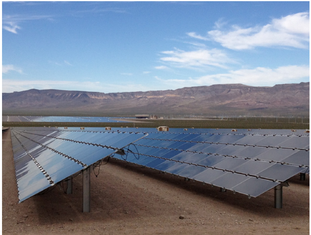
COPPER MOUNTAIN 2 Solar Photovoltaic project in Boulder City, March 2013.
